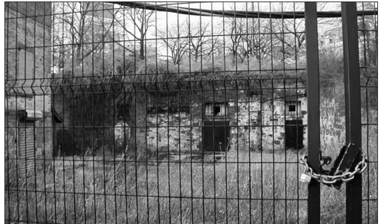
These granite masonry vaults were built in the 1870s to store kerosene and other volatile lamp fuels that replaced costly whale oil. Photo by Ernest Busch
